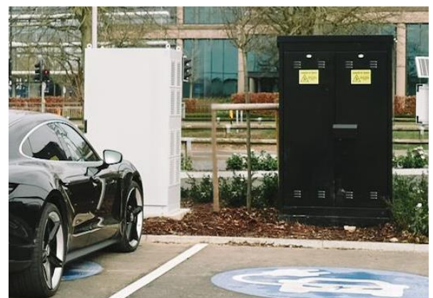
Figure 3 – RMC 1250 Cabinet housing car charging equipment. EV charging station 150kW at Westgate Retail Park, Slough (Osprey Charging).
