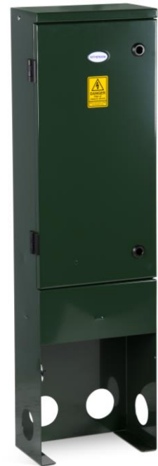
Figure 1 – RH300 Feeder Pillar
