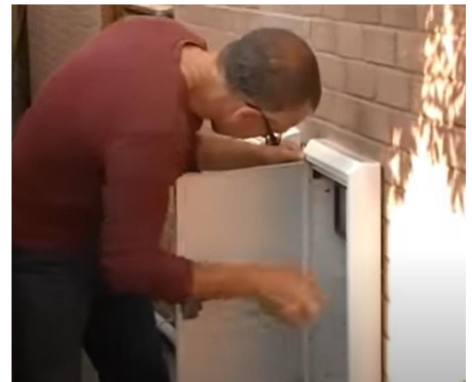
Figure 2 - Fitting an R17 door and frame into place over a GRP meter box
